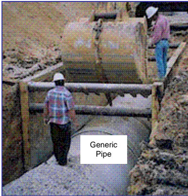
Collection system pipe sizes range from 8-42 in diameter.
