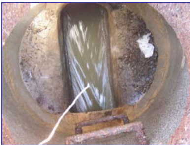
Flow measurements are taken throughout the collection system to determine the correct pipeline size.
